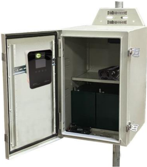
UPL 2 Battery System
