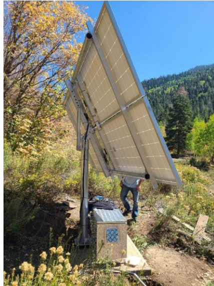
Assembled Solar Array
